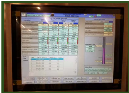
SCADA application secured by CyberLock
